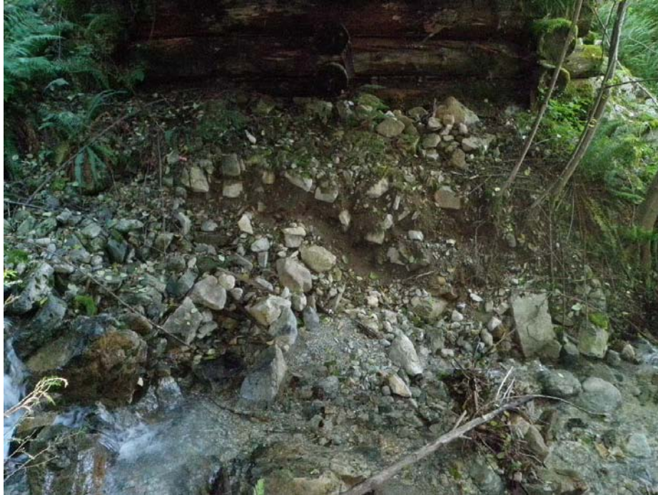
Town abutment scour
