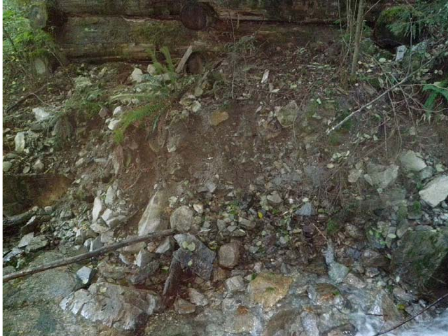
Woods abutment scour
